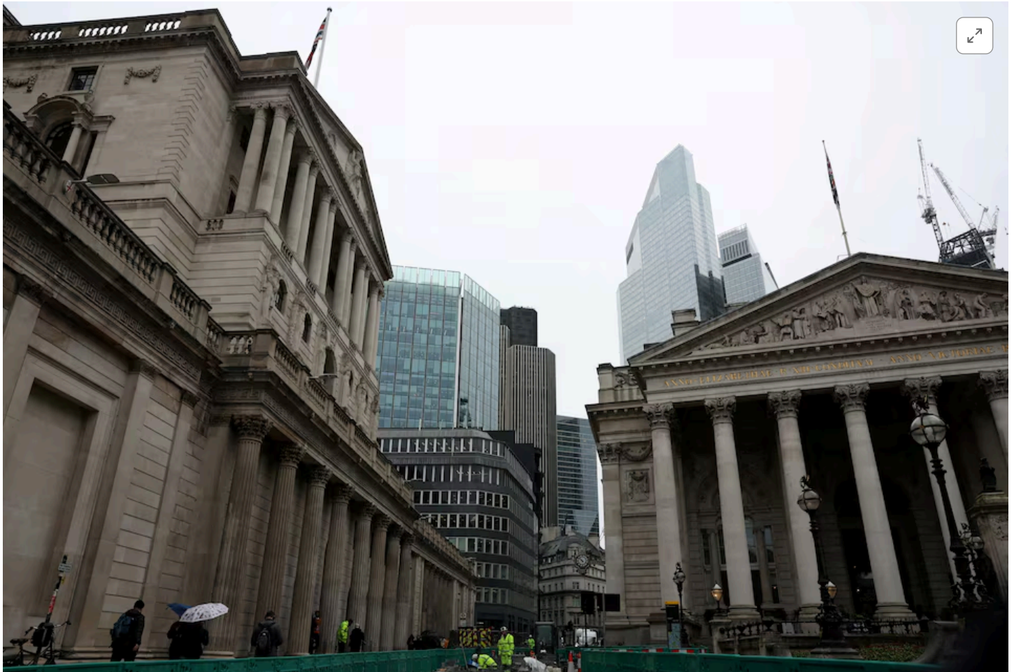
[1/2] Road construction workers carry out work outside the Bank of England in the City of London financial district in London, Britain, February 13, 2024. REUTERS/Isabel Infantes/File Photo Purchase Licensing Rights
